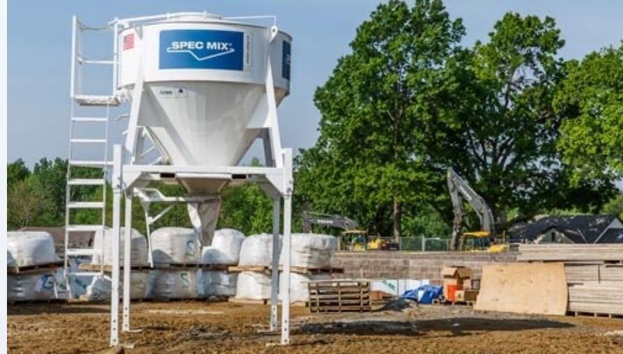
Mortar Storage Silo
