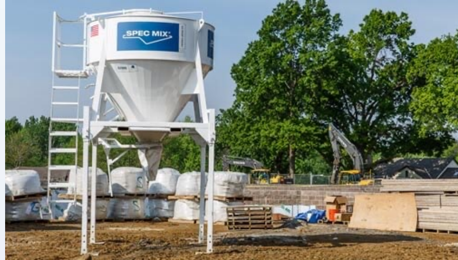
Mortar Storage Silo
