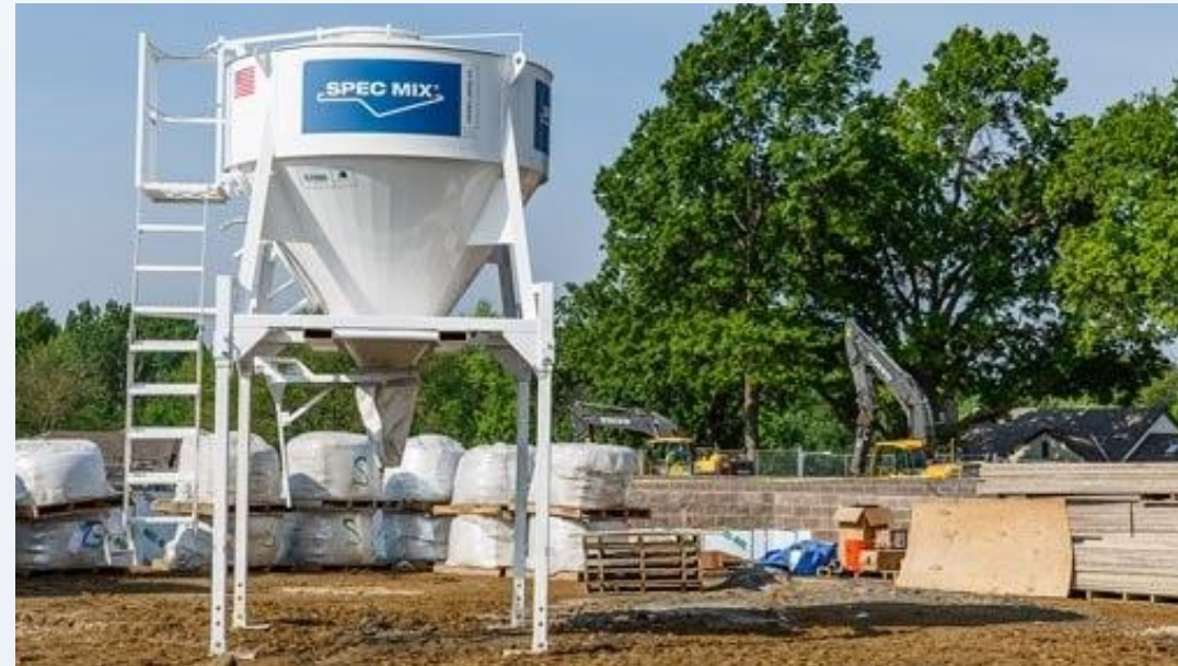
Mortar Storage Silo
